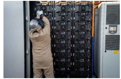
Swoose I 9.9 MW, 19.8 MWh
