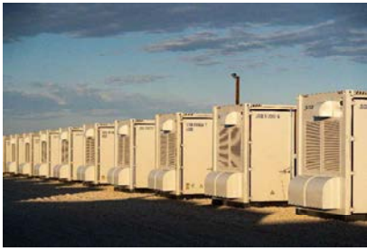
Crossett 200 MW, 200 MWh
