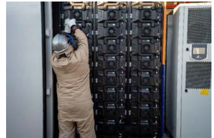
Swoose I 9.9 MW, 19.8 MWh
