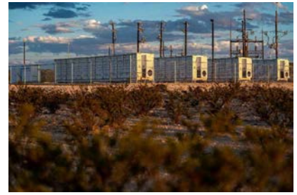
Swoose II 100 MW, 200 MWh
