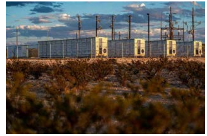
Swoose II 100 MW, 200 MWh
