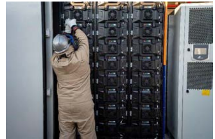
Swoose I 9.9 MW, 19.8 MWh
