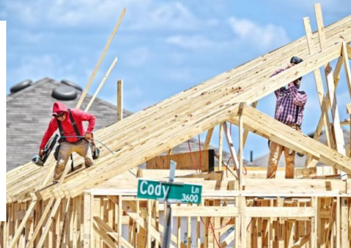
Construction workers frame a house Tuesday at the corner of Cody Lane and Doris Drive, in north Denton. A new state law limits what cities can do to regulate construction materials used by homebuilders.
