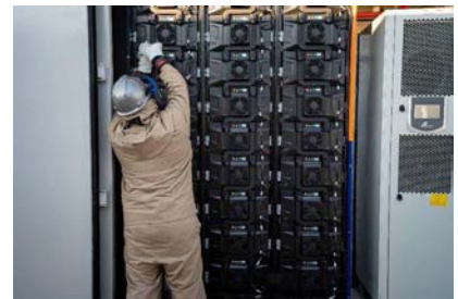
Swoose I 9.9 MW, 19.8 MWh
